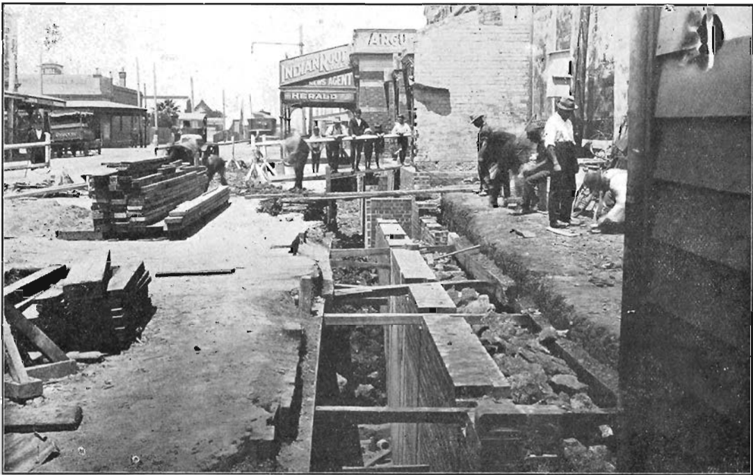
Retaining walls being built on the west side of Victoria-street. The street is to be lowered 13 ft. to allow traffic to pass under the new line.
