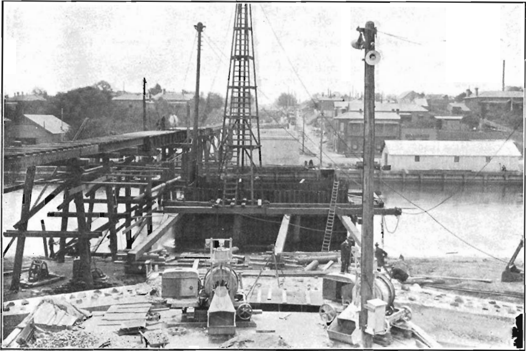
Looking over the Maribyrnong River Bridge towards Bunbury-street. Pier No. 1 is in the foreground.
